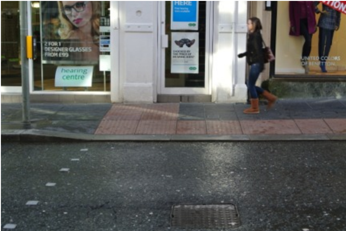
Picture 8: The benefits of an improved controlled pedestrian crossing in Derry are reduced by locating the control box too far from the tactile paving.
